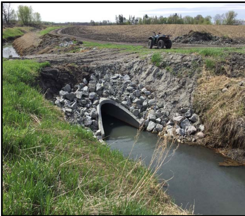
Right: ROB map for Stearns CD 11 Bottom: Culvert replacement and protection during the Stearns CD 11 repair.
